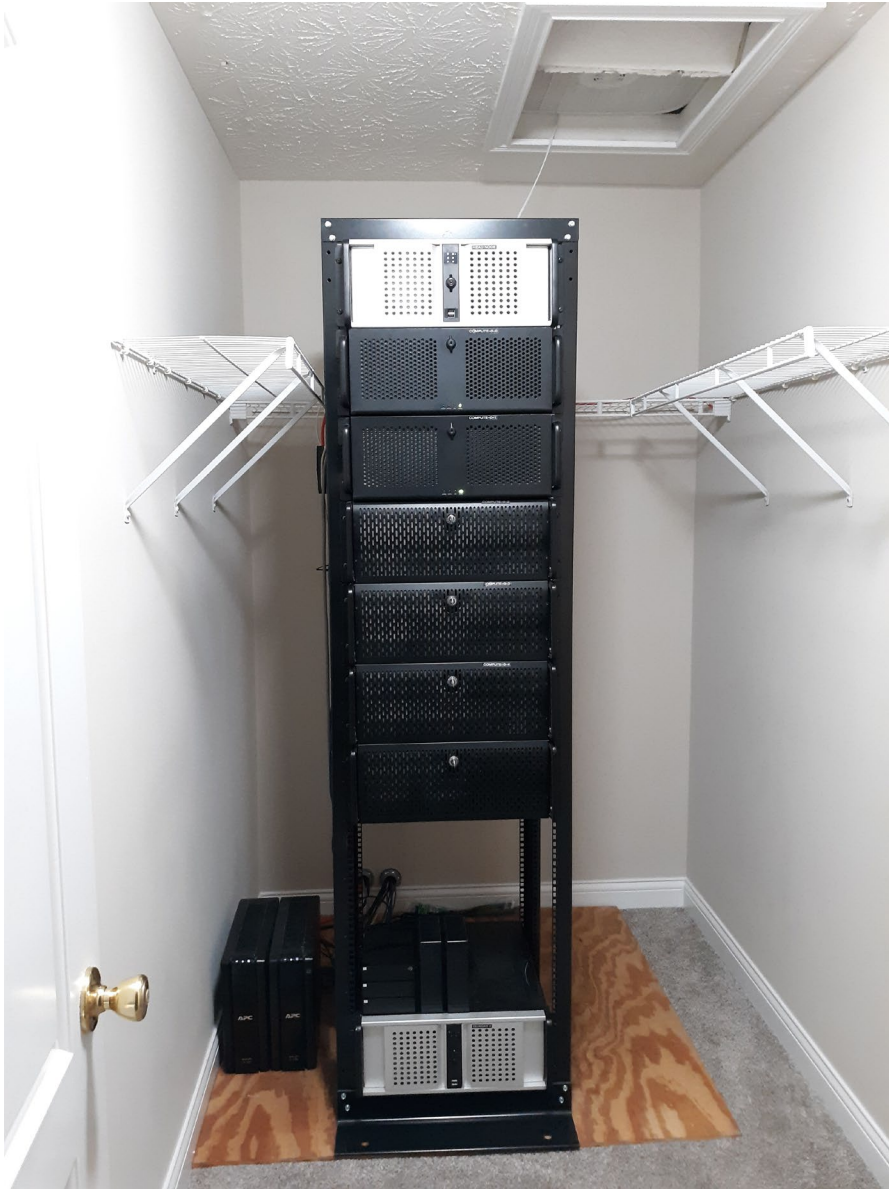
Figure 79 – HPC Clustering Rack, Workstation, Cooling, UPS Units, and Wireway
